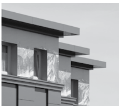
Long-term renewal and maintenance with cost-effective modernisation using ALUCOBOND®: Höxterstraße in Hagen, Germany
